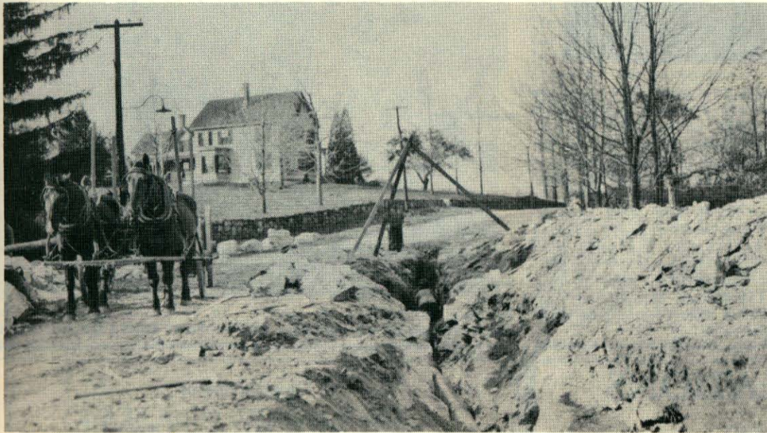
Laying water pipes, 1913, on High Street, Center Section, when town water system was being installed.
