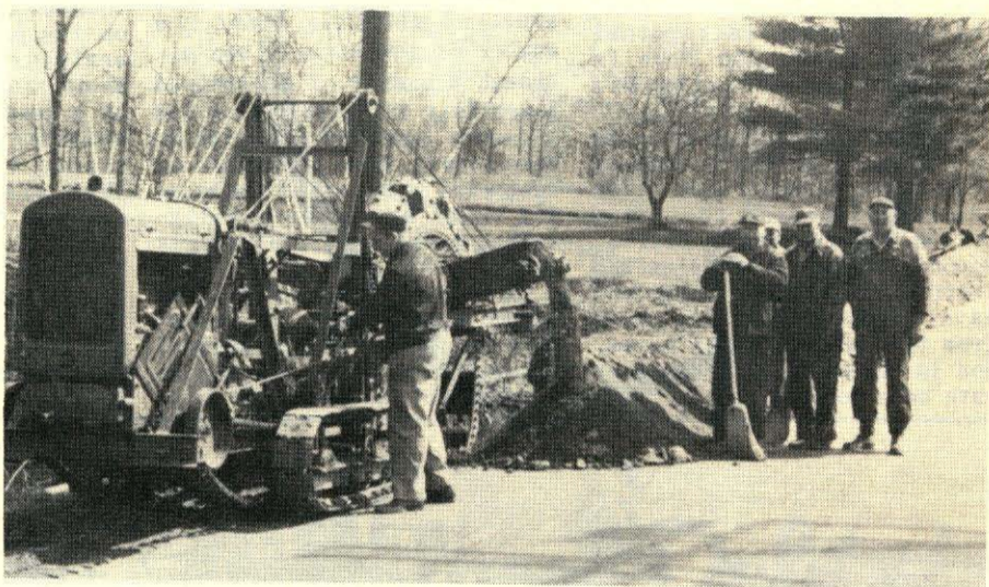
Lowell Gas Company street department crewmen lay a section of main in Chelmsford. This town is among the fastest-growing in the Commonwealth.
