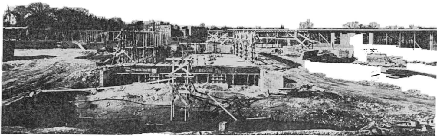
NEW SCHOOL CONSTRUCTION MOVES AHEAD---This panoramic shot show graphically the progress to date in the construction of the new Center school being erected off Billerica street. High school buildings may be seen in center background.
