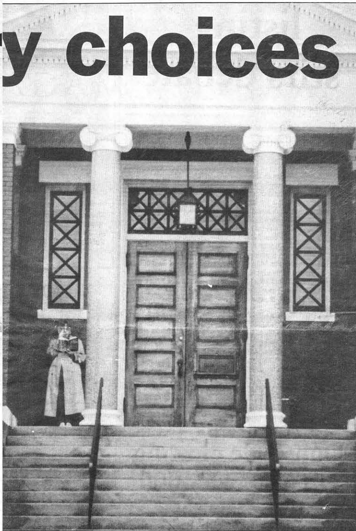
TOUGH CLIMB — Officials acknowledge they must make the Adams Library above accessible to library users who are handicapped. (Photo by
