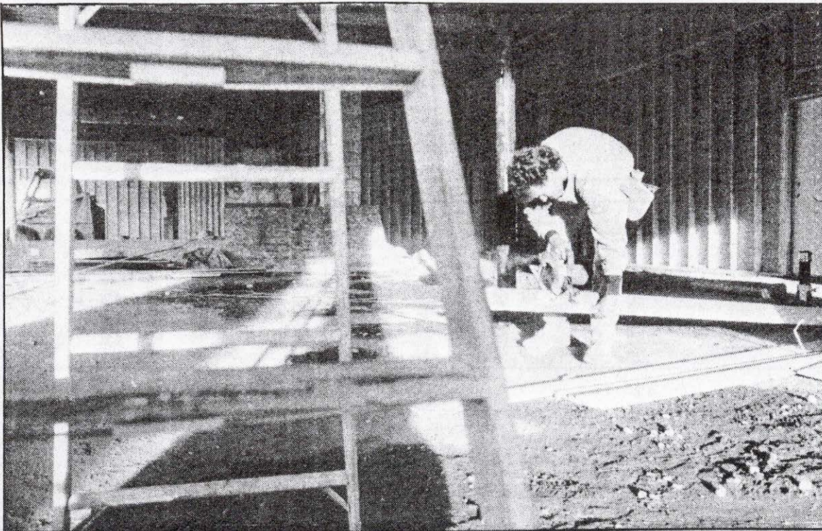
TOM LYNAM of Chelmsford nuts clapboard Tuesday for an exterior wall of Centre Mall, which is being rennovated for seven retail businesses. (Staff Photo by Marc Holland)
