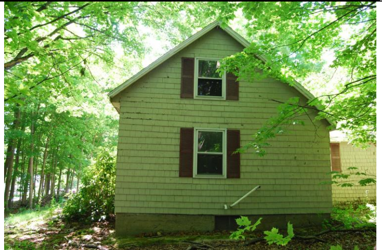
View looking southeast toward side (north) elevation of main block. Note extended roofline and rear addition at right side of elevation. Ell partially visible at far right.
