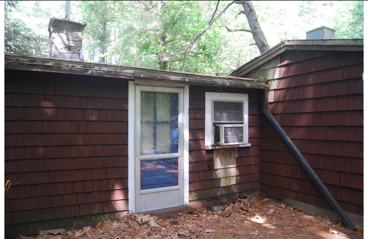
View looking northwest. Door and window at north end of east elevation. Ell at right.
