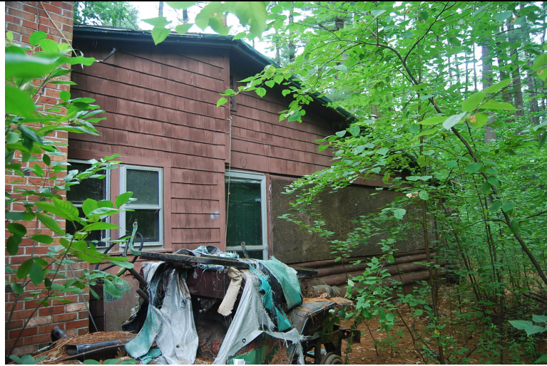
Photo 7. View looking north at southeast elevation of addition. Possible undercut porch at right.
