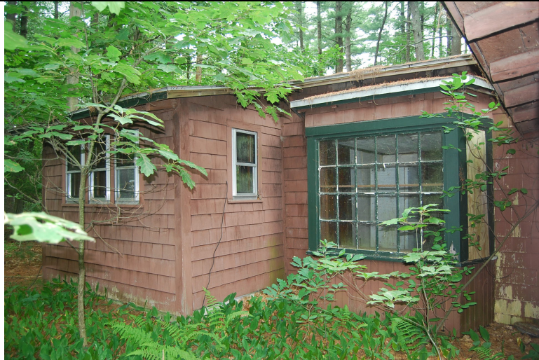
Photo 6. View looking north at projection and bay window. Log cabin partially visible at right edge of photograph.
