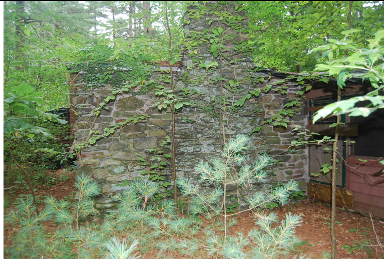
Photo 9. View looking southwest at stone wall with integrated chimney located at east end of addition. Screened porch partially visible at right.
