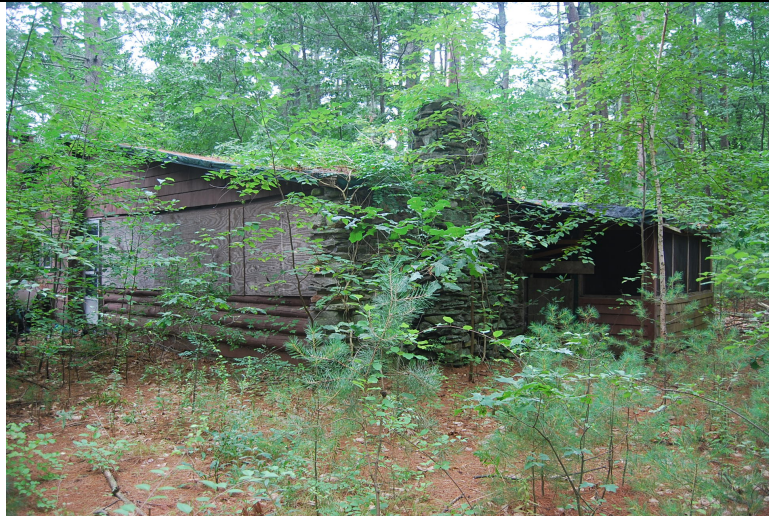
Photo 8. View looking west at east end of addition. Undercut porch at left. Large chimney wall at center. Screened porch addition at right.
